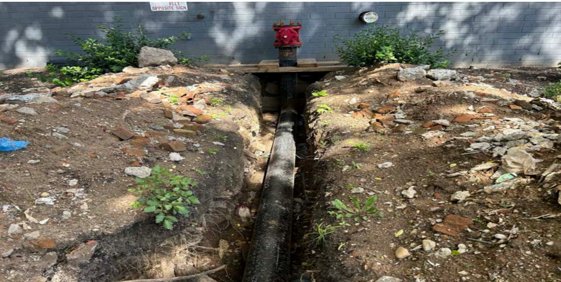
Figure 88. The interstitial spaces that occur on all sides of these pipes between the earth and common building utility laterals are among the most common areas of rat/mouse harborages (and with sewer laterals –entry) in urban areas and building perimeters—especially if there are penetration points at the foundation that are not sealed correctly with the right materials, or they break down over time. Moments before taking this photo, a rat was seen carrying a big piece of food and disappearing into some mystery cavity where the pipe connects to the building (next photo).
