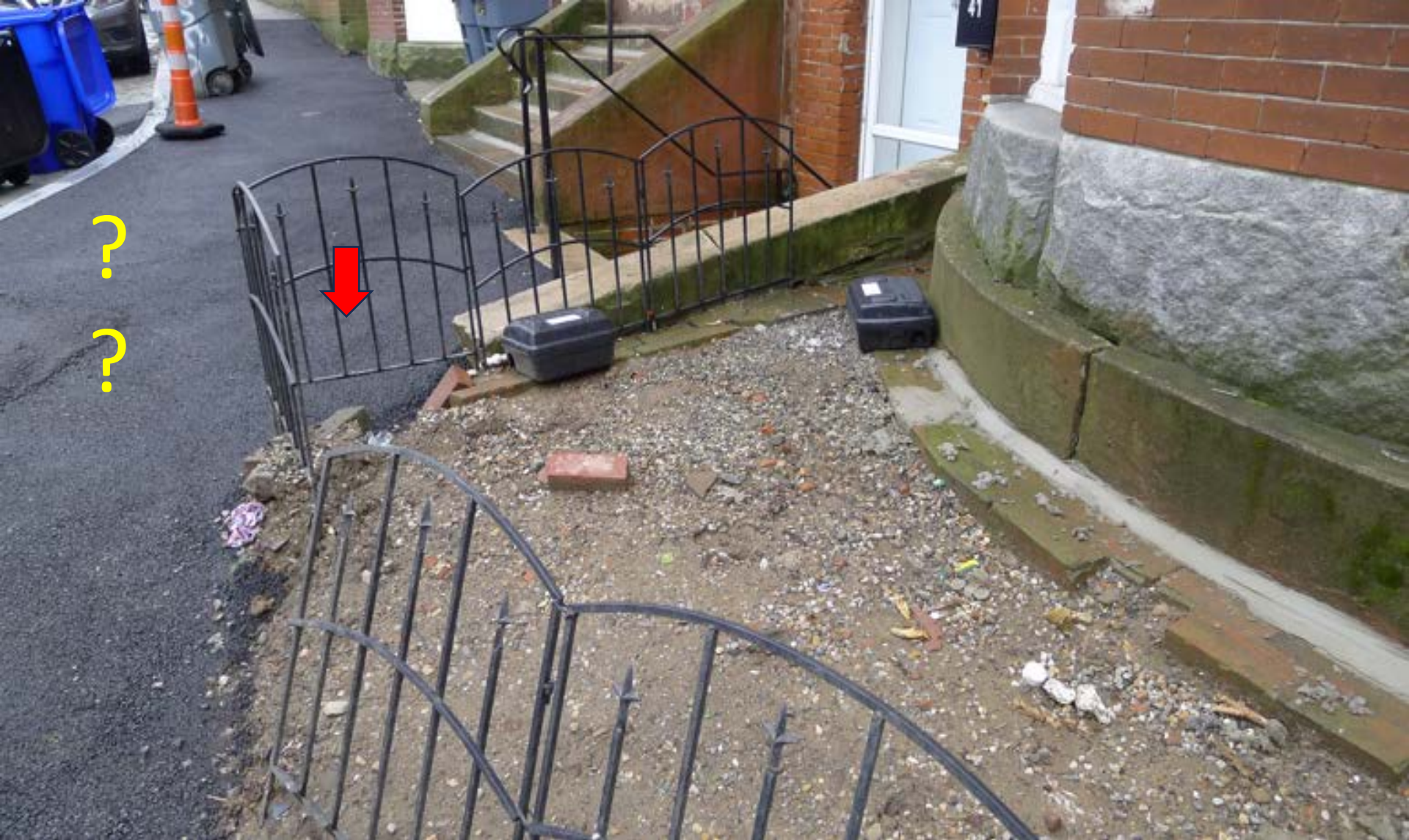
Figure78. Roxbury had severe rat infestations in nearly all areas visited. Note this yard and the sidewalk (and multiple bait stations trying to fight off the rats). The rats have burrows already constructed beneath the new asphalt (red arrow). How much of this entire new asphalt sidewalk is due to previous rat burrowing/destruction?
