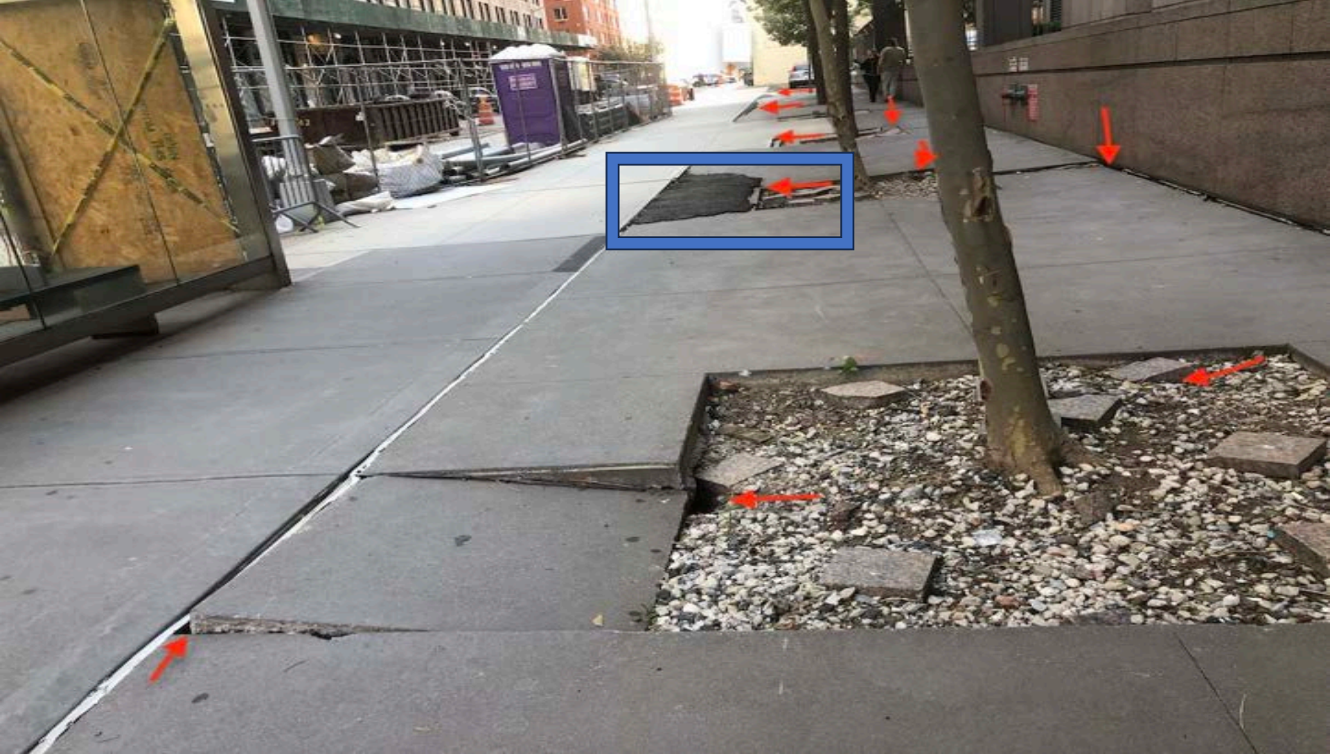
Figure 84. Sidewalk and retaining wall dismantling by one block's Norway rat colony. Each of the 10 red arrows points to an entire sidewalk panel undermined by rat tunnels running below. If rat burrows are not intercepted quickly, their tunneling destruction proceeds over months, not years. Note the all-too-common asphalt patch repairs (blue box) which never last for very long and are aesthetically unpleasing as well as presenting a tripping hazard to pedestrians. Damage costs for city Departments can run into the millions. (Photo: Corrigan, 2023) New York City.
