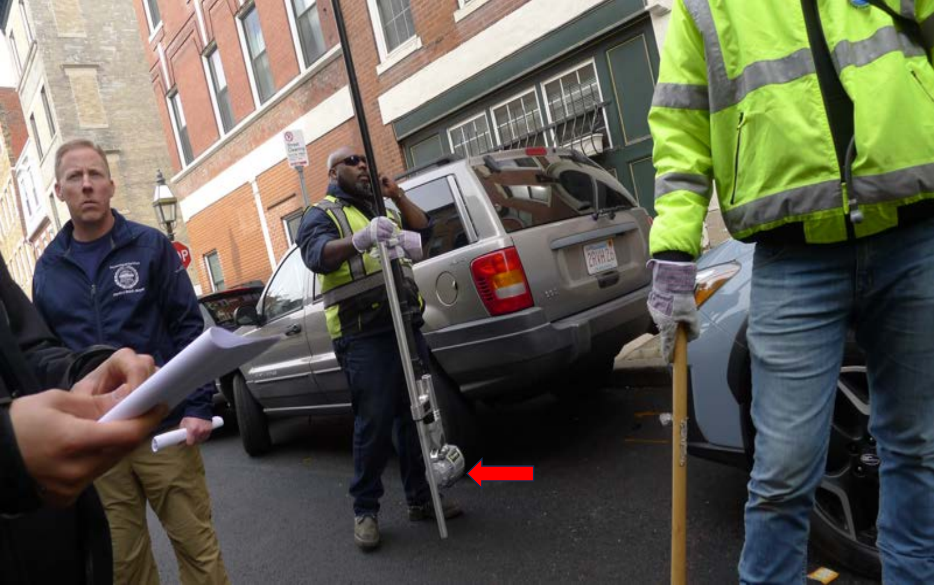
Figure 65. The BRAP team accompanied the Boston Water and Sewers group to several areas of Downtown as selected by the rodentologist (only certain sewers are vulnerable to rats). The DWS teams pulled those manholes and inserted special cameras (arrow) down into the sewers for the BRAP team to view sewer structures and observe for the presence or absence of rats in those everyday street sewers.
