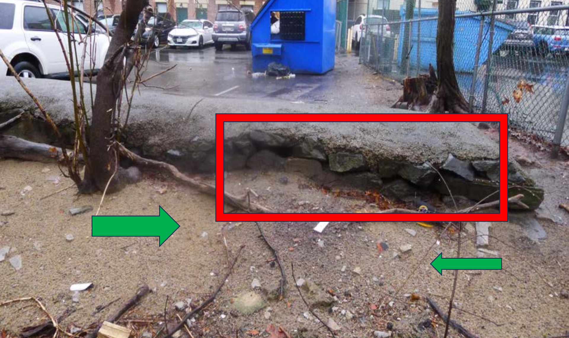
Figures 80-81. A closer viewpoint of the dumpsters with spilled and overflowing food trash. This retaining walls is being completely dismantled by the rats burrows (Red box). All the soil (green arrows) is a result of rats excavating the support fill out of the wall. Eventually, this wall will collapse should a car “nudge it” while backing into one of the allocated parking spots on the other side.
