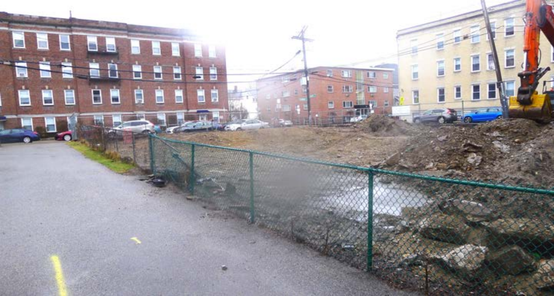
Figure 87. Pre-demolition and/or earth moving construction sites should always be surveyed for established rat presence prior to the demo-construction event. The blind practice of placing out bait boxes at a construction site rat-sighting unseen just as tangible practice would not control any rats should they in fact be present. (A very worn city rat myth). The one bait box installed along this fence might give the impression “something” is being done to control any “disturbed rats”, but a Best Practices Protocol for Construction Site Rodent IPM needs to be included to provide true protection to the community against disturbance of any existing rats as determined via a BRAP-assessment and survey. (Roxbury MA).
