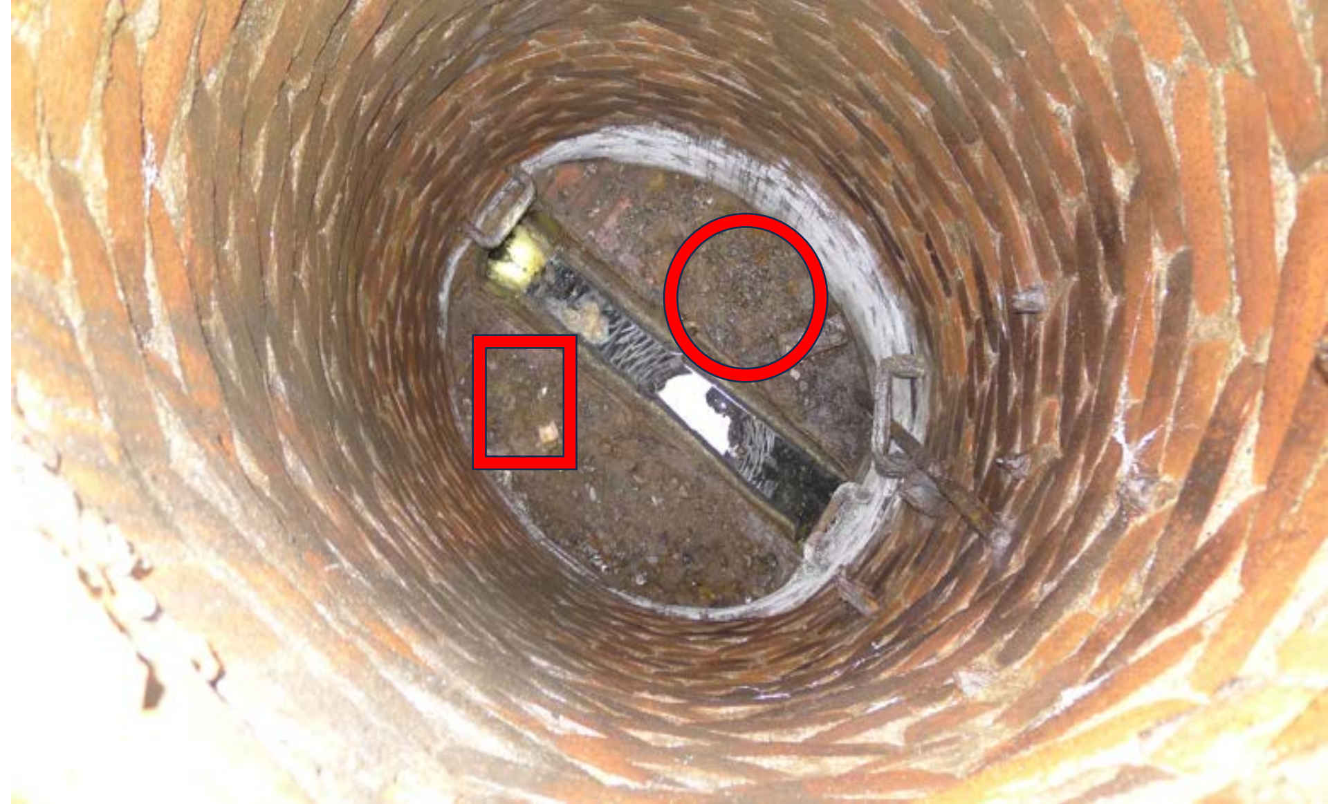
Figure 66. After pulling the manhole plate and looking down from the street level, rat droppings (within red circles) are easily noted on the sewer's ledges (similar to a stream running along through a woods, land, etc.) This ledge provides city rat managers a spot to install various types of traps and/or bait stations to assist in sewer rat control.
