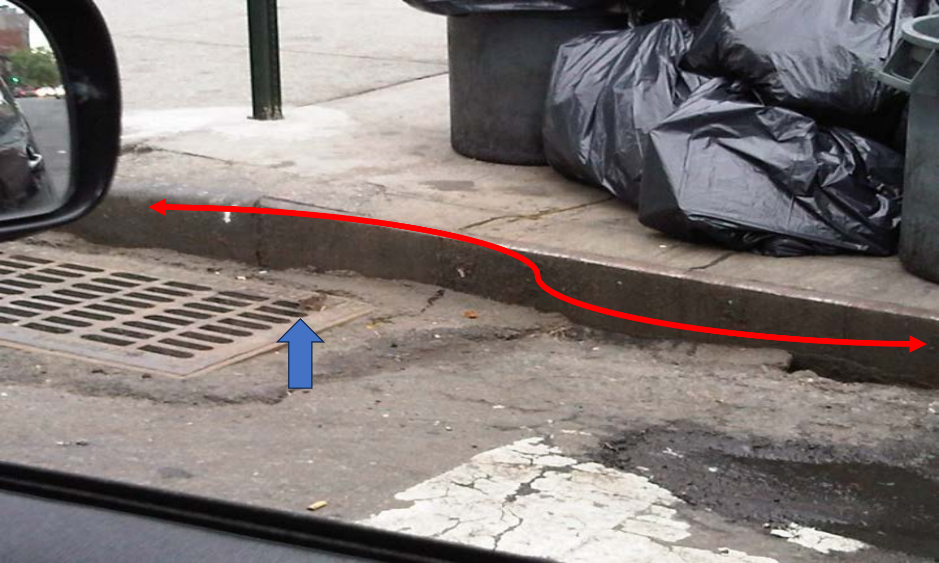
Figure 76. Very expensive sub-surface damage to the roadway, the sidewalk, the curb, and the associated drain basin which has been repeatedly repaired due to rat tunnels year after year. Notice the rat waiting to scurry to the food trash bags. This rat is the tip of the rat-berg below. (Corrigan, 2021, NYC).
