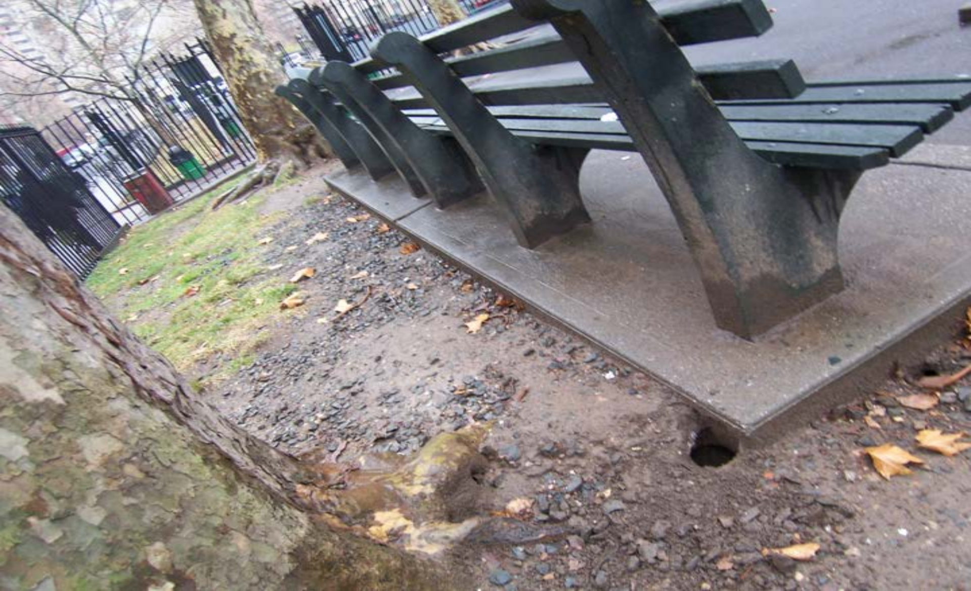
Figures 83-84. Norway rats prefer to locate their burrows and nests below heavy objects for the protection such provides (cement slabs of all types, roads, sidewalks, boulders, etc.). Rat burrows remove the support fill and soil for the infrastructure resulting in stress cracks and/or eventually the collapse of the infrastructure. If left unaddressed, these park benches will be significantly compromised and will require expensive repairs and/or replacements. (A recent NYC park bench).
