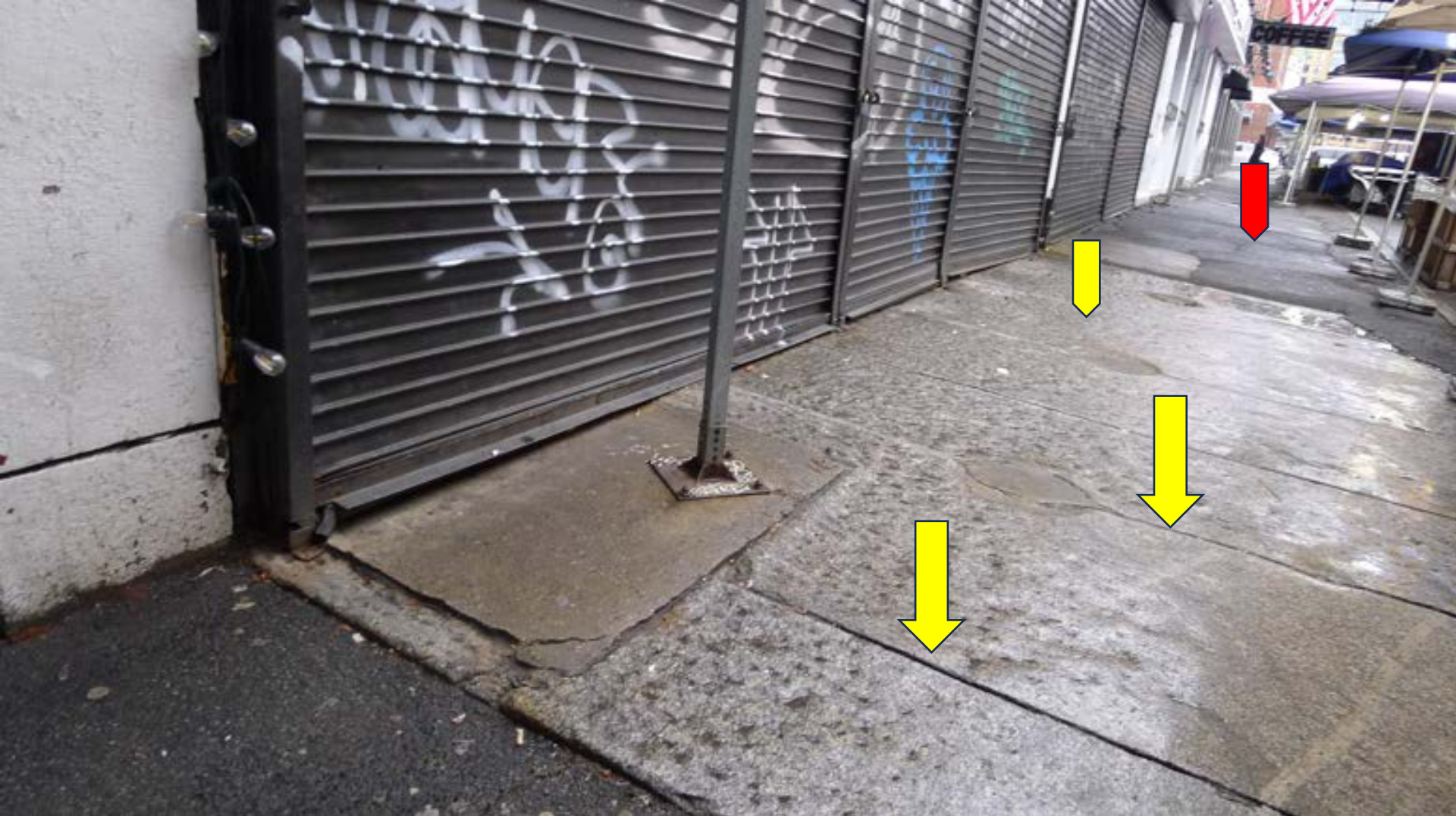
Figure 32. The importance of rodent proofing to avoid expensive city repairs. Note the mix-mash of sidewalk elements over time. All this patchiness creates many interstitial spaces for the burrowing rat—especially in areas where food odors and food drops, fragmentation of food, etc. is so highly pervasive as in the Haymarket. All such sidewalks must be examined expansion-joint-by-expansion-joint for integrity and to ensure the correct sealants are used to deny rats entry to the sub-surface creating additional voids that will need patches and expensive repairs (red repairs)
