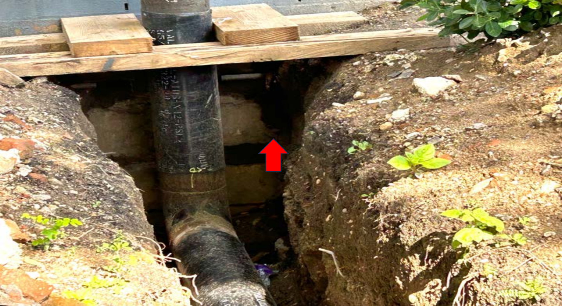
Figure 89. A moment before I took this photo, a large, old rat, in broad daylight, carrying a large piece of food disappeared into the dark hole of the interstitial spaces associated with this emergency water line. The takeaway is that construction may expose rats that were there unbeknownst to the locals all along, but construction does not “cause rats” to suddenly develop in a neighborhood that was previously free of rats. Enhanced sanitation alerts and efforts to citizens a month or two prior to any construction in any Boston neighborhood that has filed 311 complaints will have a 100X greater impact on reducing how many rats or mice are seen once construction begins. (See written report).
