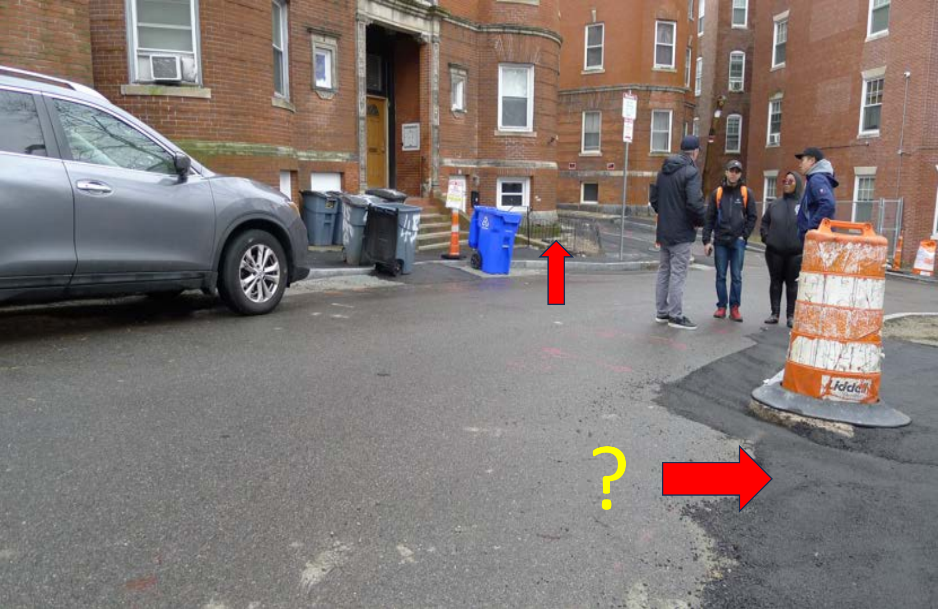
Figure 79. The BRAP team members discussing the heavy rat activity in Roxbury. Many of the sidewalks and front building foundation areas contained damaging rat tunnels and burrows.
