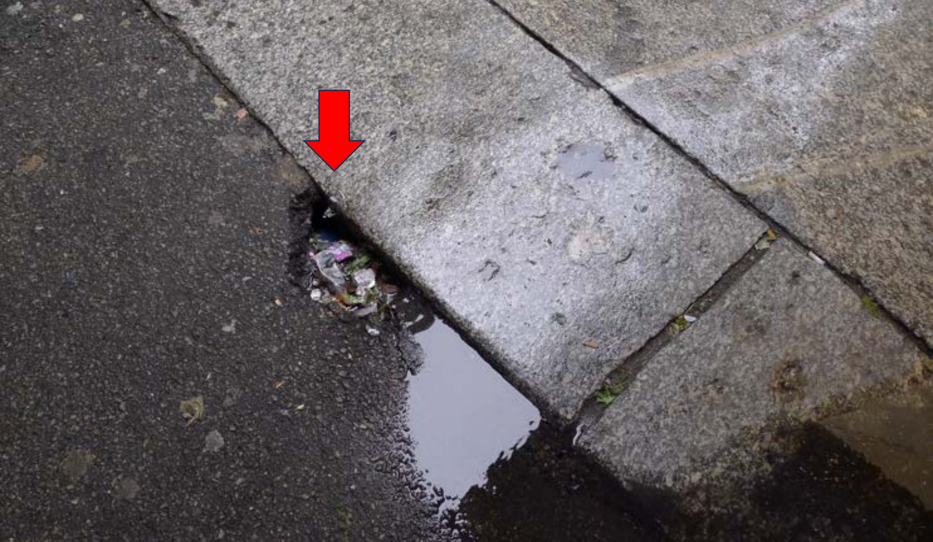
Figure 31. A very active rat burrow beneath a sidewalk in downtown Boston close to the Haymarket. Rats will completely undermine an old city's heavy granite slabs causing them to collapse and be replaced with a much less sturdy infrastructure of asphalt in addition to being much less aesthetically pleasing to the charm of old historical neighborhoods of the city. See Figures 32-35 for further discussion on the importance of keeping up with such repairs.
