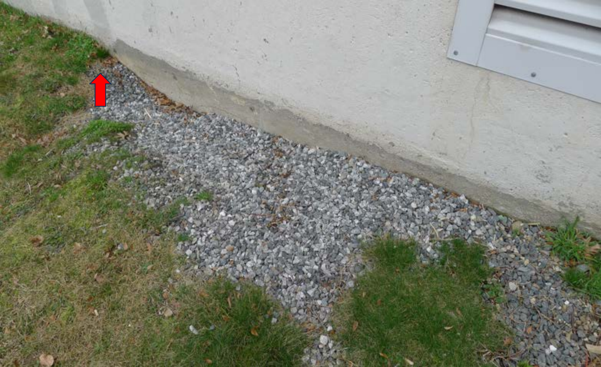
Figure 82. Large space of foundational support soil/fill removed by Norway rats and filled in with gravel by staff at a BHA building. The very industrious rat will often simply begin again at the margins of the fill (red arrow) continuing the frustration. The key is to intercept this at the very first hole when it would require a mere cave in of the one hole. Once it progresses as seen here, it becomes a laborious $$ project.
