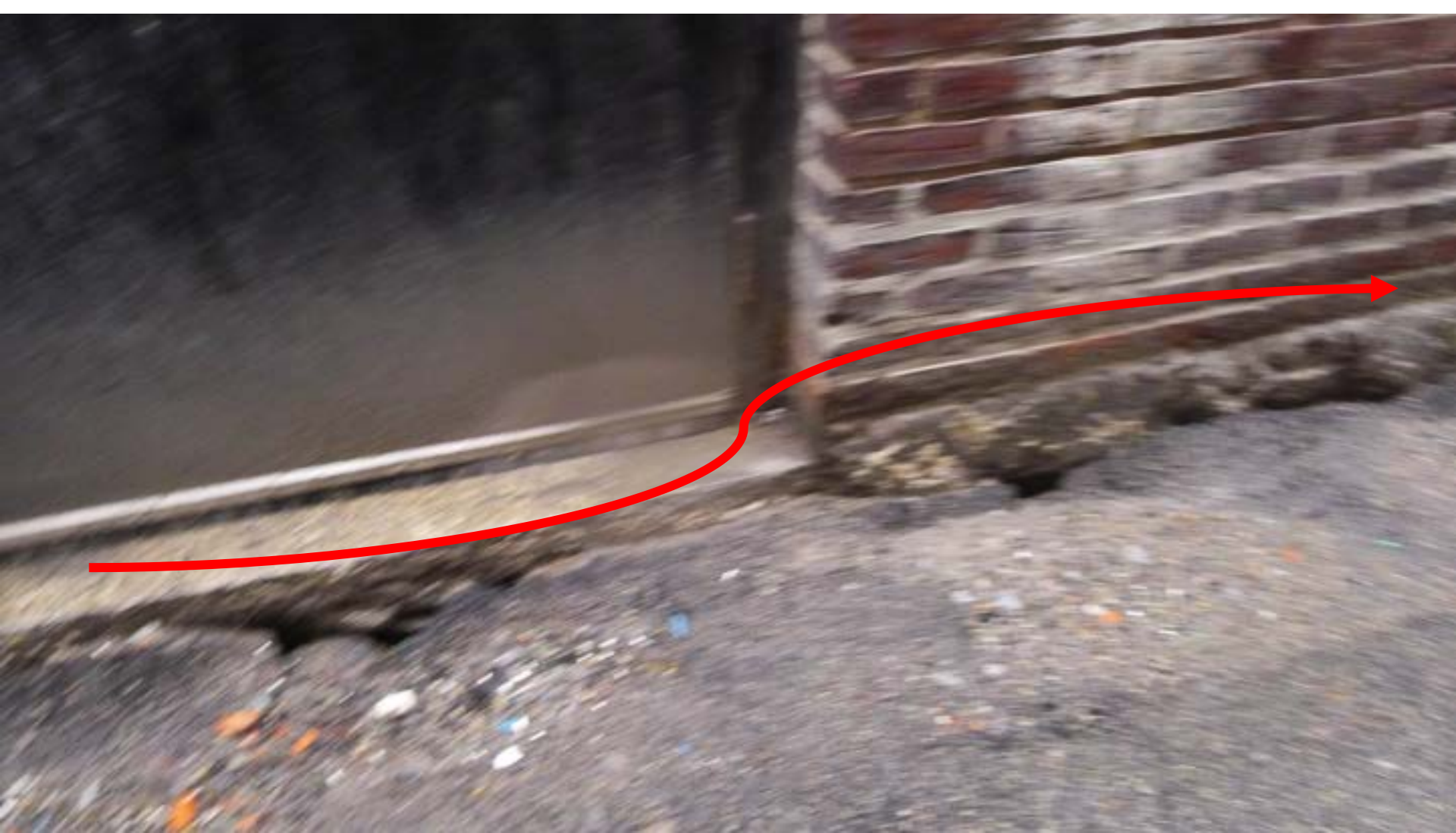
Figure 75. Within a Boston alley. A frequently noted scenario in multiple areas of Boston during the two-day field BRAP assessment. Norway rat destruction of sidewalks and building perimeters often results in serious damage to the foundations, cracking of sidewalks, basement flooding, etc., because such rat holes and cracks leads to water seepage into these areas; and during the winter the freezing channels expand blowing out walls, and other structural elements.
