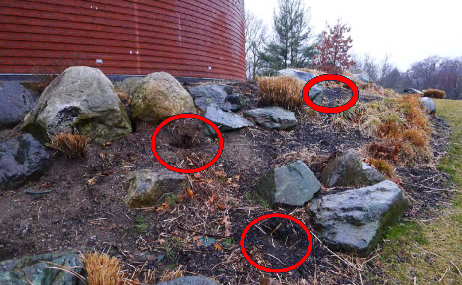
Figure 58. At Ringer Park's main entrance and community building area, these active rat burrows are a direct result of a few unmanaged dumpsters only 40 yds. across the front parking lot. (Note: rats love to establish their burrows/nests in grounds and landscapes that are sloping at the high end of the slope (assists in nature's wick-away function of keeping burrowing animals' nests dry).
